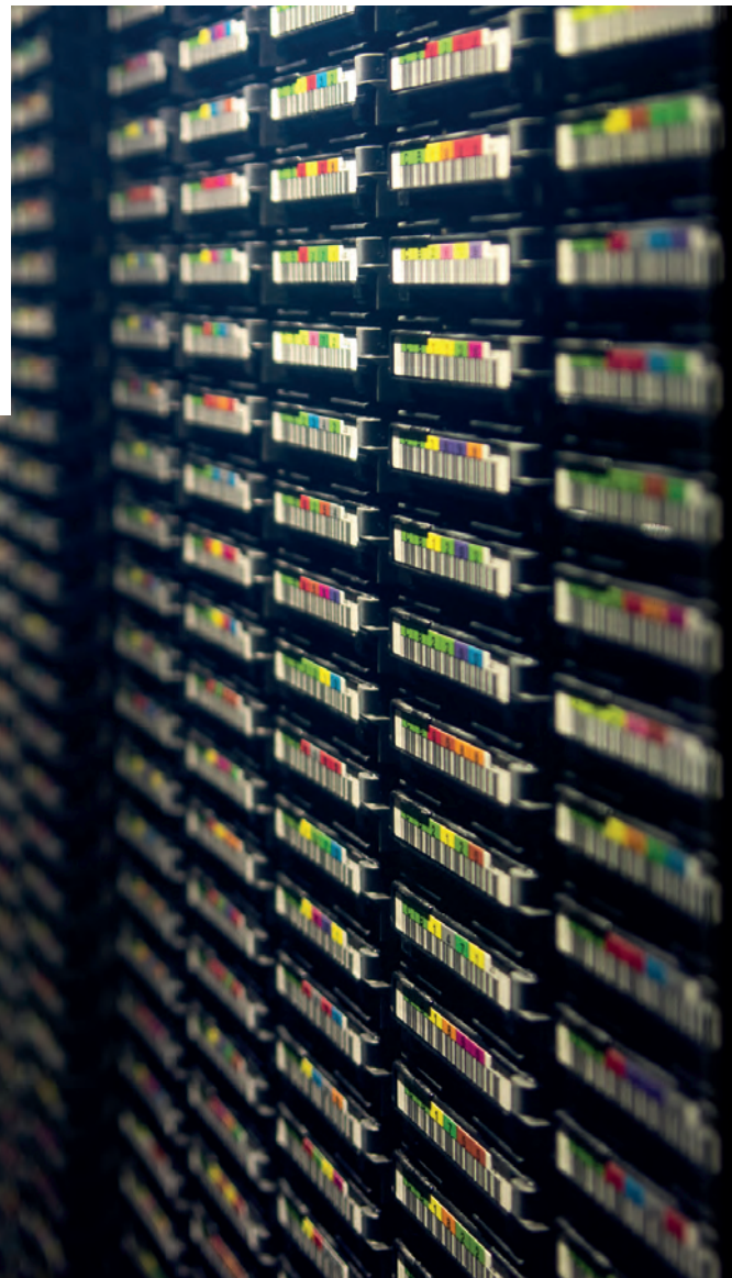
Inside of the tape library
