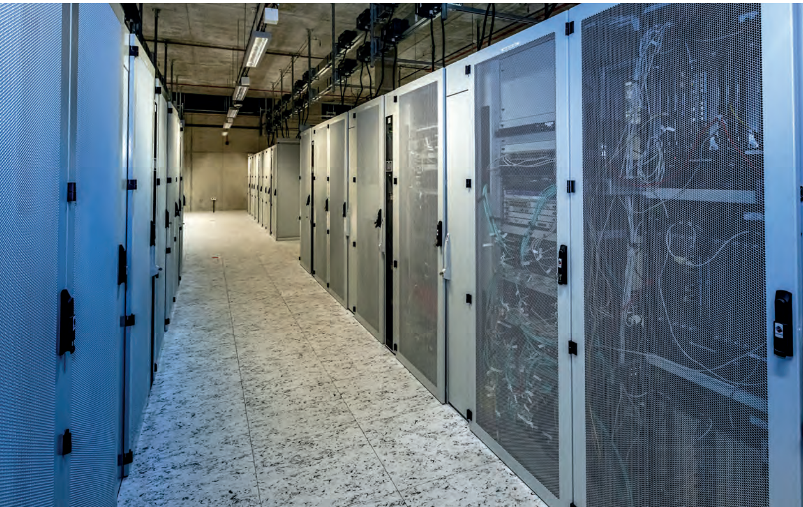
The Data Center infrastructure in PSNC
