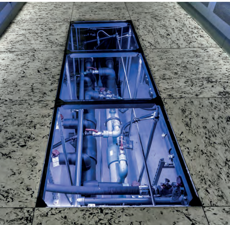
The cooling infrastructure in the PSNC Data Center
