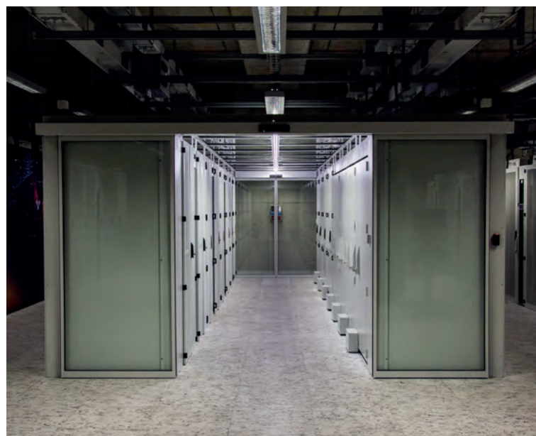
Data infrastructure facilities in PSNC
